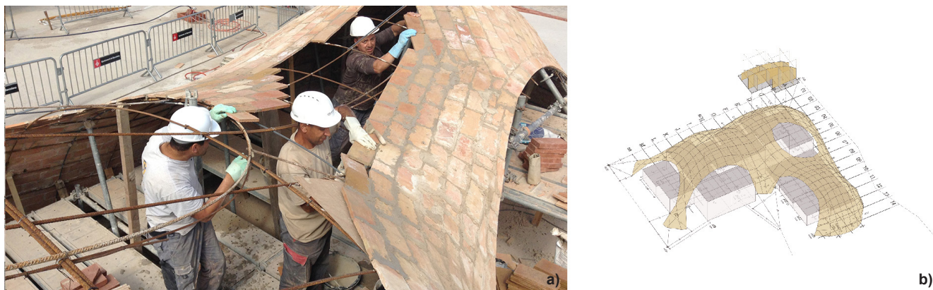
Figure 6. “Brick-topia”, Map13 Barcelona, 2013, a) under construction (Photo: Manuel de Lózar & Paula López), b) falsework scheme.
