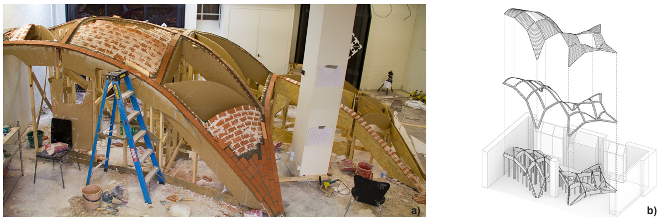
Figure 7. Workshop at MADA, Melbourne, 2013, instructed by P. Block (ETH Zurich), J. Bellamy (Re-vault), T. Schork (MADA) and D. Van Horne (Grimshaw Architects), a) under construction, b) exploded 3D showing the falsework and construction scheme.
