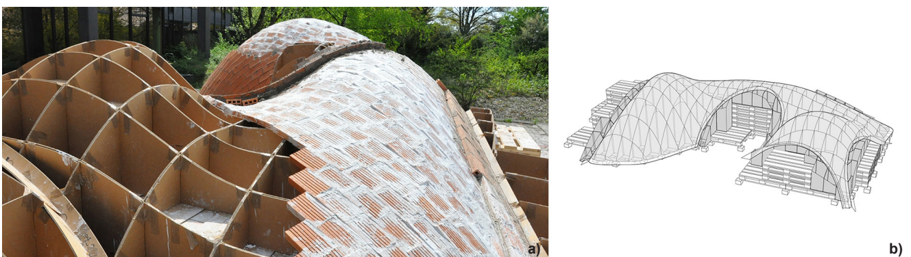
Figure 5. First free-form tile vault. BRG, ETH Zurich, 2011, a ) under construction, b ) falsework scheme.
