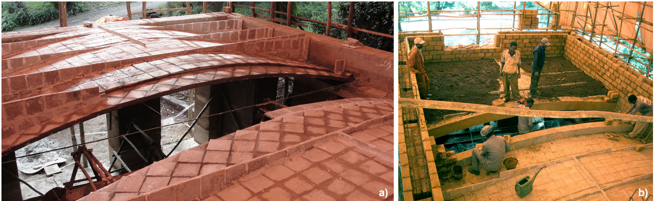
Figure 8. Tile vaults at SUDU project, BRG, ETH Zurich, (2010-2011), a) tile vaults with lightweight stiffening walls, b) tile vaults with lightweight stiffening walls and compacted fill.
